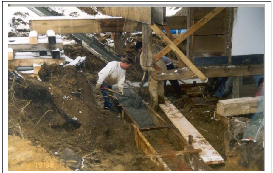
Concrete footings were poured and a cinder block foundation added under the 1810 ell.
